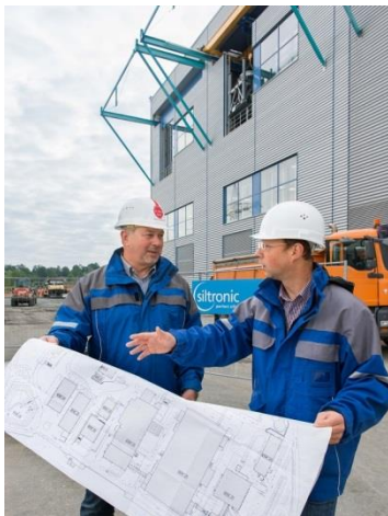
Siltronic project manager Johann Sperl (right) und Wacker Chemie project leader Gerhard Ofenmacher (left) in front of the new Siltronic pulling hall in Freiberg
